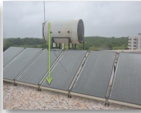
Solar Water Heater
